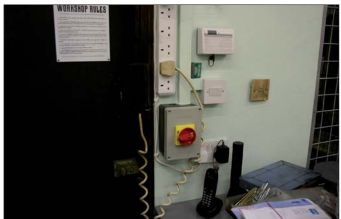
The Master switch by the exit.
