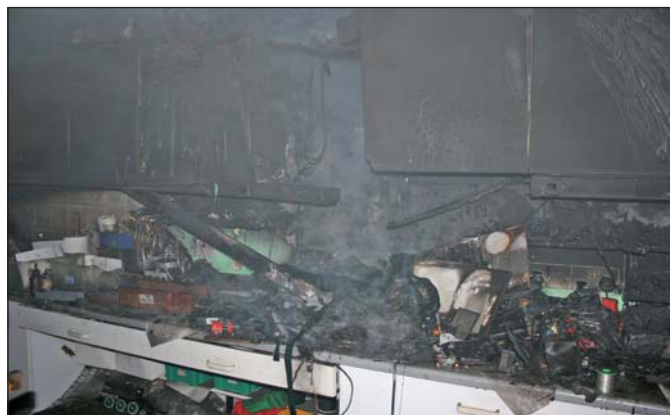
Some of the fire damage.
